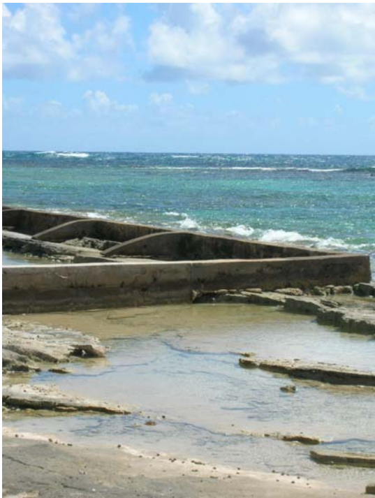
Remedial action through the construction of a breakwater was necessary to address the effects from both sand mining and Hurricane Luis along Sile Bay.
